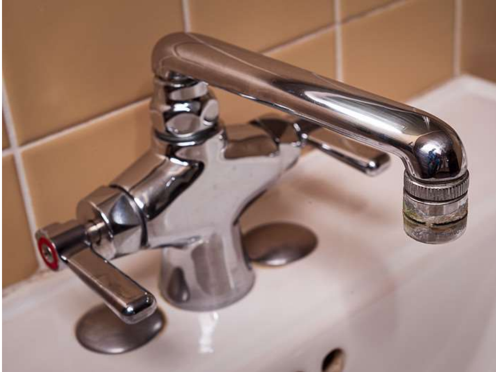
Figure 3: Leaded fitting on a sink faucet (photo credit: US EPA/ORD)
